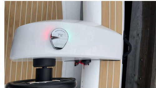
Installed nav lights
